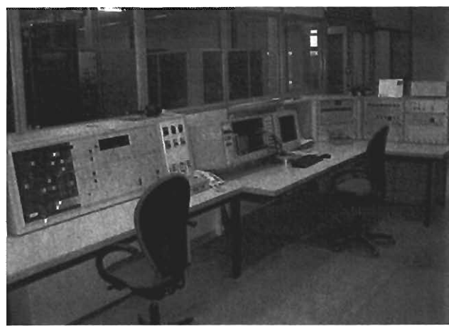
Control station for tests up to 15kA
